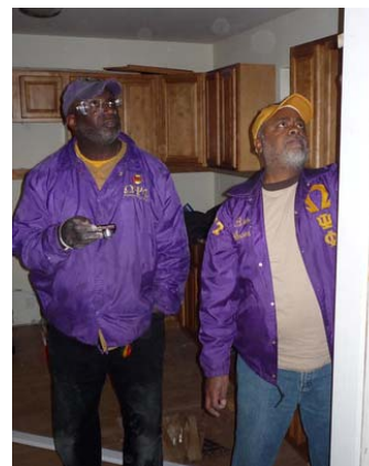
Bros. Gerald Massenburg ('77 Rho Zeta) and Mitchell Sharp ('03 Nu Nu) make minor repairs.
